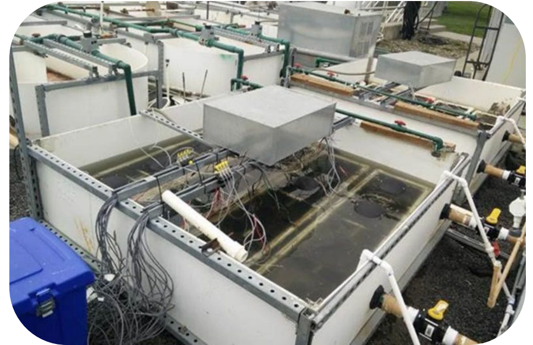
MFC wastewater treatment pilot system at Washington State University
